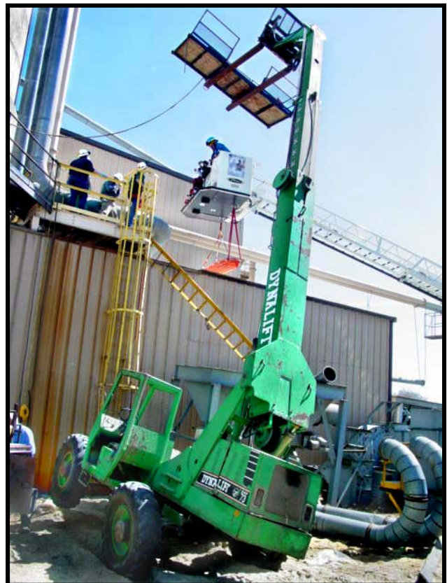
Photo 1 – Police photo of the scene showing the new catwalk, and the boom forklift, leaning to the right.
