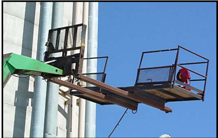
Photo 5 – Shot from underneath the platform showing the extended steel channels attached to the forks of the machine.
